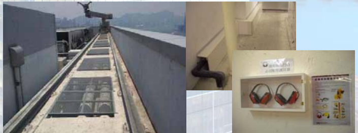
Safety Mesh and Safety Equipment can reduce accidents and the Shield Boards can protect the facilities against water damage
