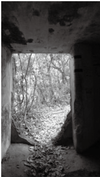
Figure 61: The emergency exit inside the tunnel. The damaged wall covered the lower half of the entrance originally. The upper half may have been covered by bricks before which could be broken through easily (Photo by author in 2010).
