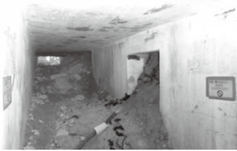
Figure 52: Tunnel connected to Regent Palace Hotel. The first entrance to the “hotel” is clearly visible in front. The second entrance is further behind with considerable damage on the roof and mostly filled up. Note the remains of the cable cover marked a black line on wall (Photo by author in 2010).
