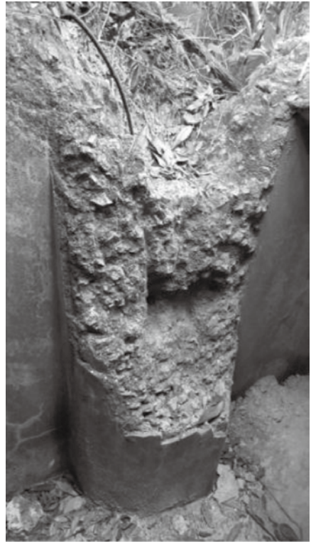
Figure 59: Inside of bulge structure. The end of a steel rebar was anchored inside the damaged hole in the bulge. Damage possibly caused by scavengers breaking open the concrete to get the steel rebar inside. Note the concrete of wartime military structure contains a lot of rock A thin layer of fine concrete covered surface to give it a smooth finish (Photo by author in 2011).
